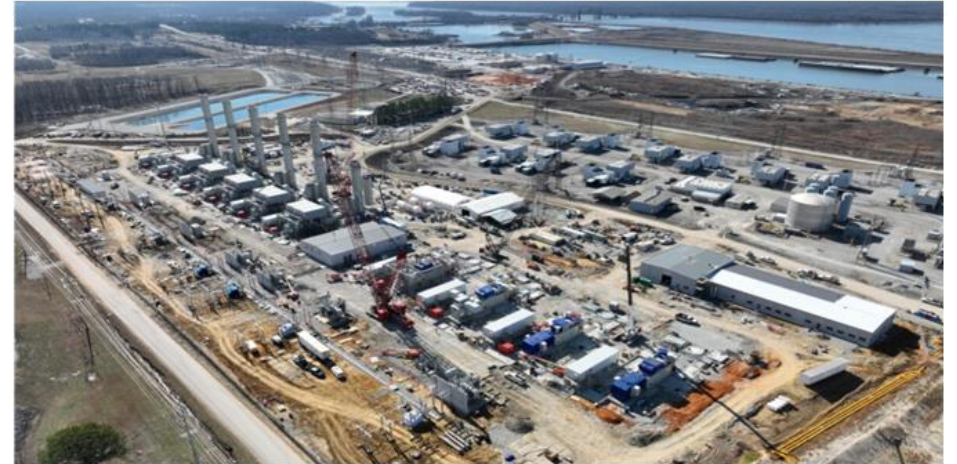
Johnsonville Aero derivative Combustion Turbine Project
