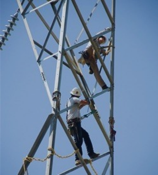
Provide affordable, reliable power.
