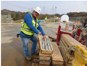
Technical Field Lead Scott Lakes examines core samples taken during drilling on the dam's earthen embankment.
