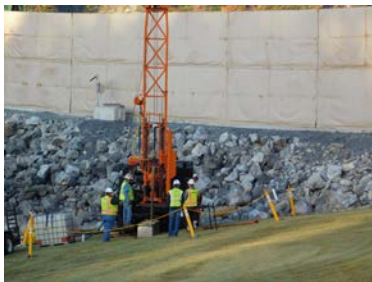
Drilling can be seen on the right rim of the earthen embankment.
