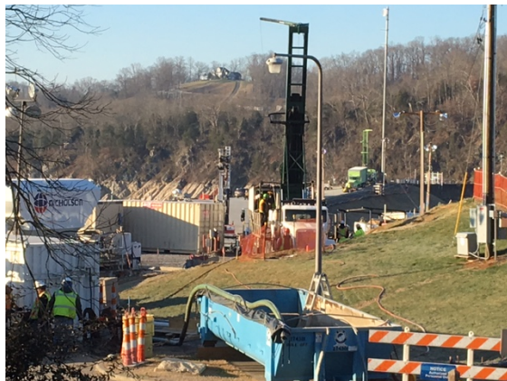
Three sonic rig drill rigs can be seen performing test operations on the earthen embankment.
