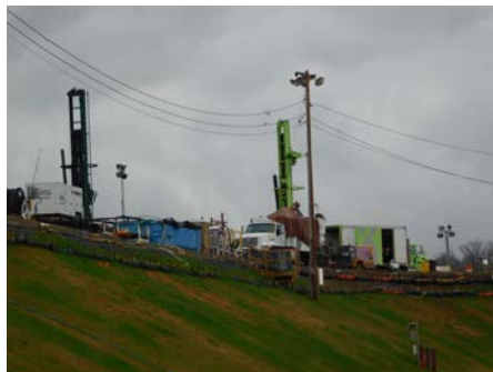
Two of the three sonic drill rigs in operation late last week. This view is from the downstream side of the earthen embankment.
