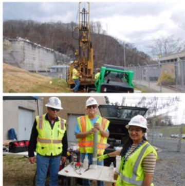
Top: Auger Drilling collects undisturbed soil samples. Bottom: Engineer Veronica Barredo points to the Shelby Tube Bill Butler is holding. Lenny Peterson, at left, checks for quality.
