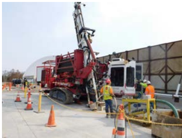
Grouting rigs on top of Boone Dam's earthen embankment are now injecting high mobility grout into the dam's smaller cracks in the bedrock.
