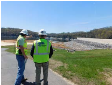
Construction manager Kevin Holbrook and Site Supervisor Jack Stanhope review the location of the future upstream berm construction. The work, which will take place this summer, will be visible to passing boaters and our Boone Dam neighbors.
