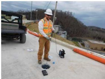
Dam Safety Inspector Matt Duke monitors subsurface conditions at Boone Dam from one of the newly installed inclinometer locations.
