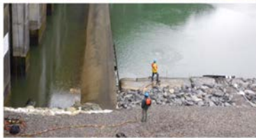
Top: Auger Drill is moved into place on platform on dam’s earthen embankment via remote control (held by worker at left).
