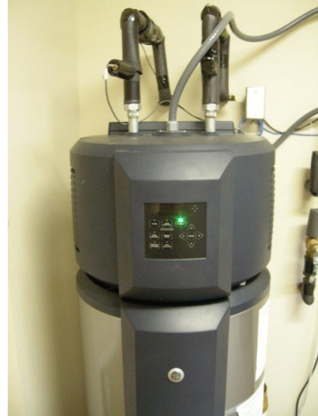
Fig. 1. GE Geospring HPWH at CC2.
