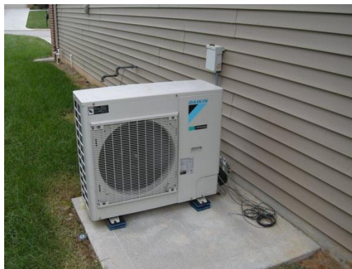
Fig. 3. The Daikin inverter compressor at CC3.
