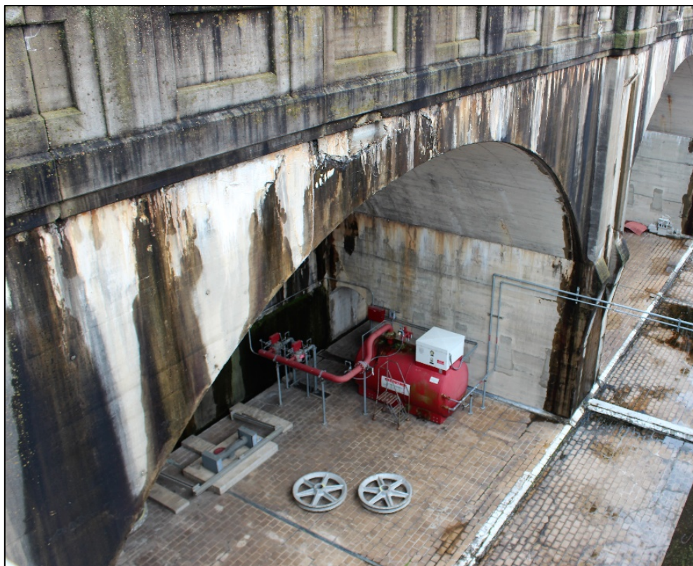
Concrete Arch Showing Spalling and Efflorescence
