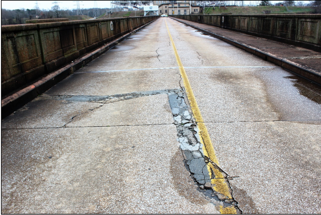
Bridge Deck Cracks
