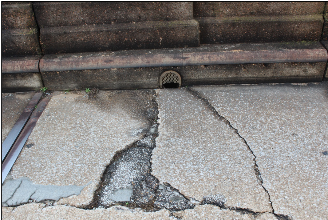
Bridge Deck Cracks
