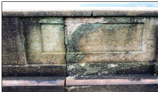
Deterioration of Parapet and Curb
