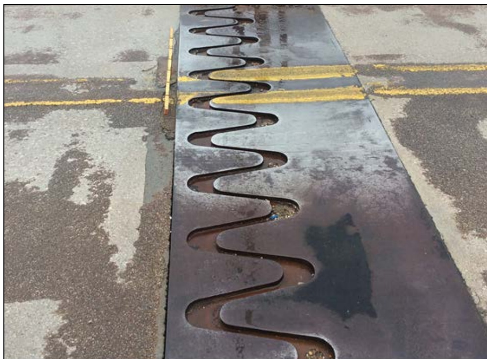
Failing Epoxy Overlay and Deteriorating Bridge Joint on Fly-over
