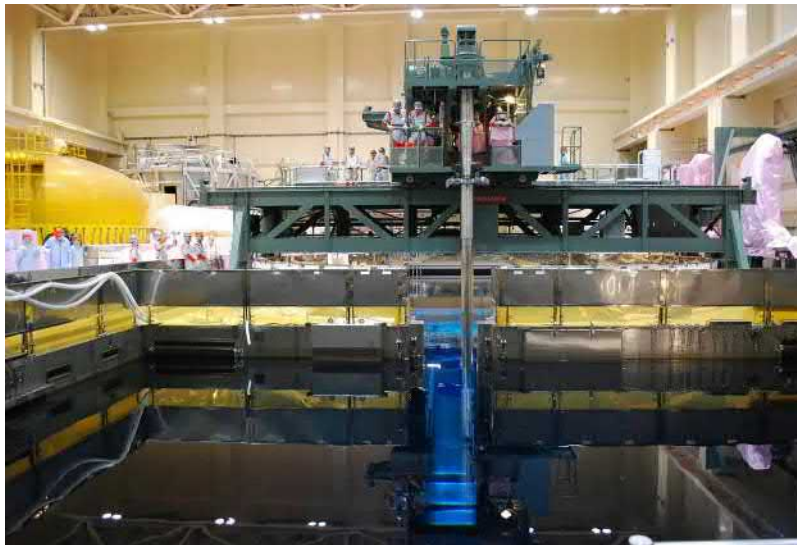
A fuel storage pool in the Fukushima plant reactor building. Surrounding this and reactors like it is a containment vessel, the last line of defense if cooling fails. Jiji Press/Agence France-Presse — Getty Images
