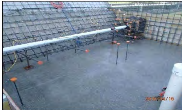
L 17C Lift 5 clean up prior to the start of the pour
