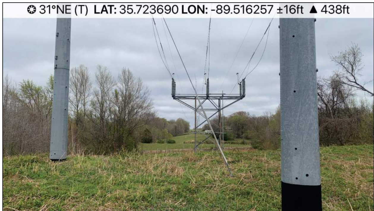
Photo 6 Facing northeast, electrical transmission towers.
