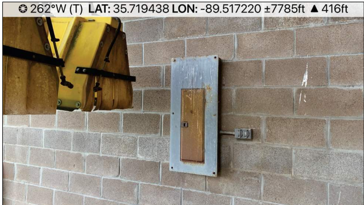
Photo 12 Electrical box inside farm storage building.
