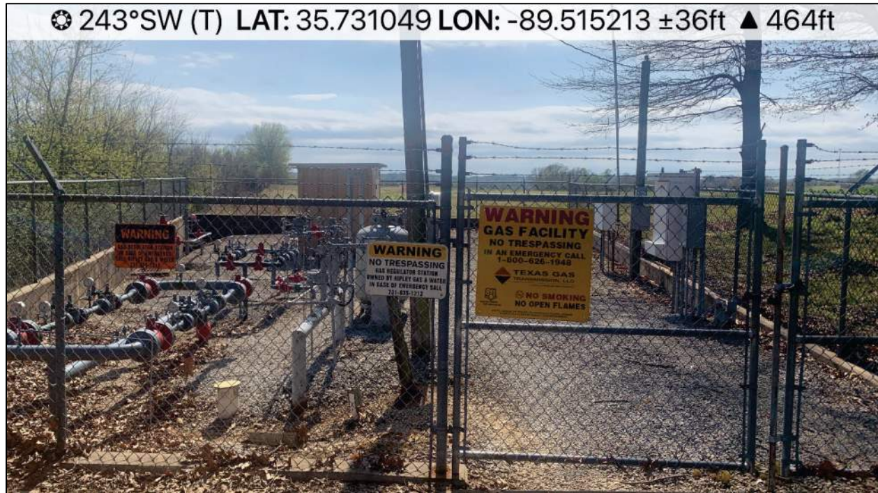
Photo 29 Facing southwest, natural gas metering station northeast of the Subject Property boundary.
