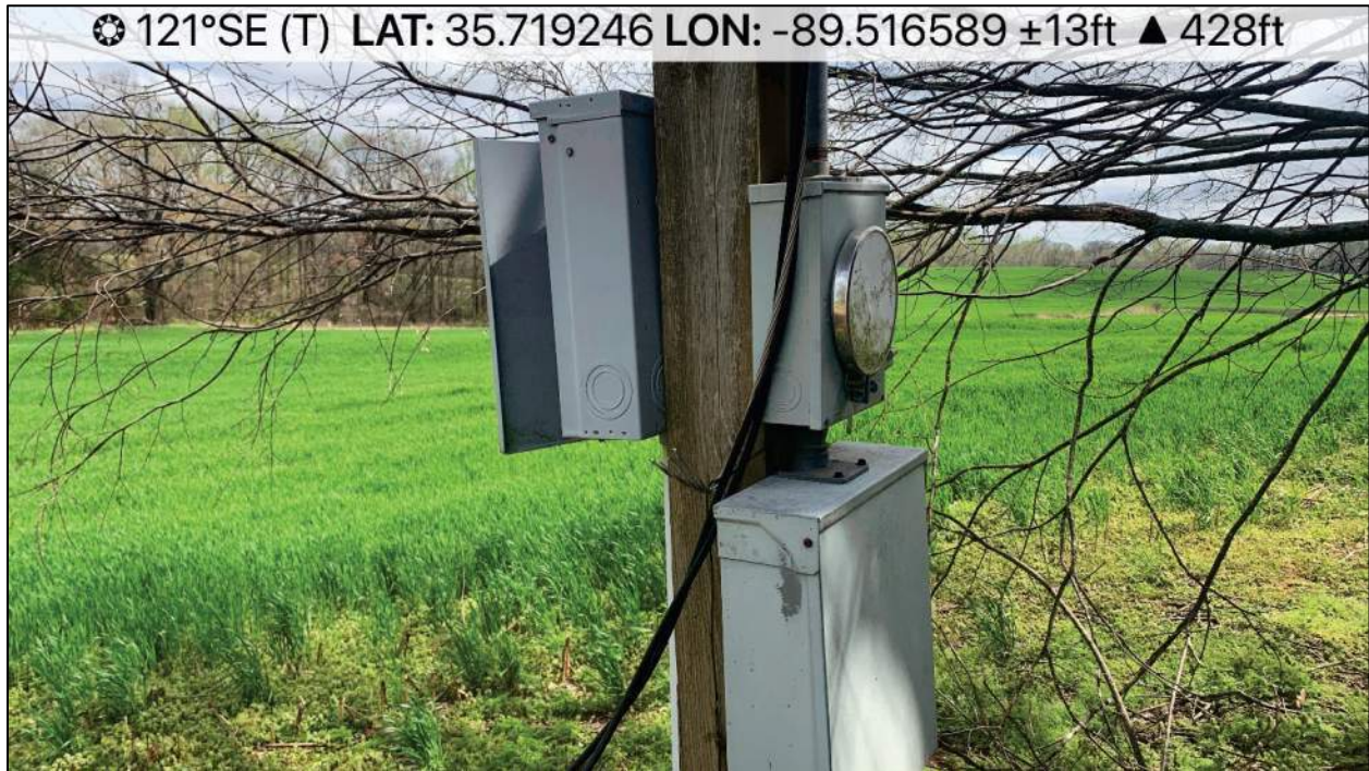
Photo 19 Facing southeast, electrical utility boxes behind silos.
