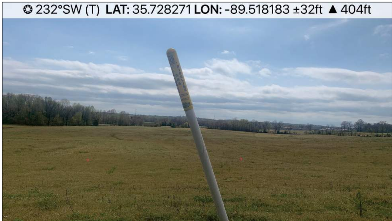
Photo 26 Facing southwest, natural gas pipeline marker.
