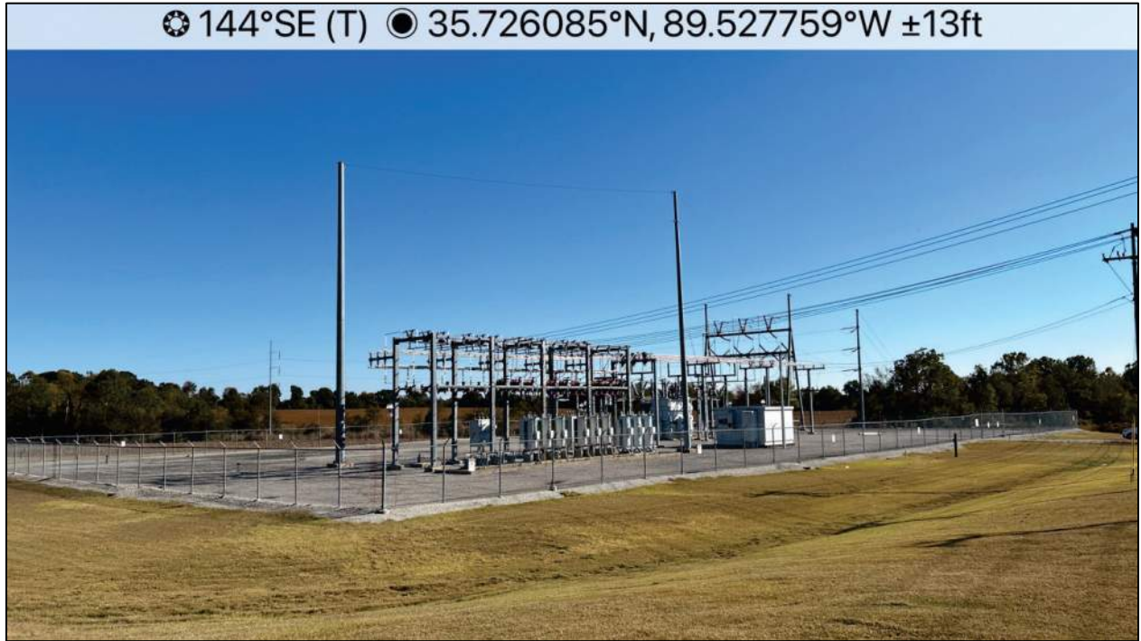
Photograph 7 – Electrical substation southeast of parcel, view southeast.
