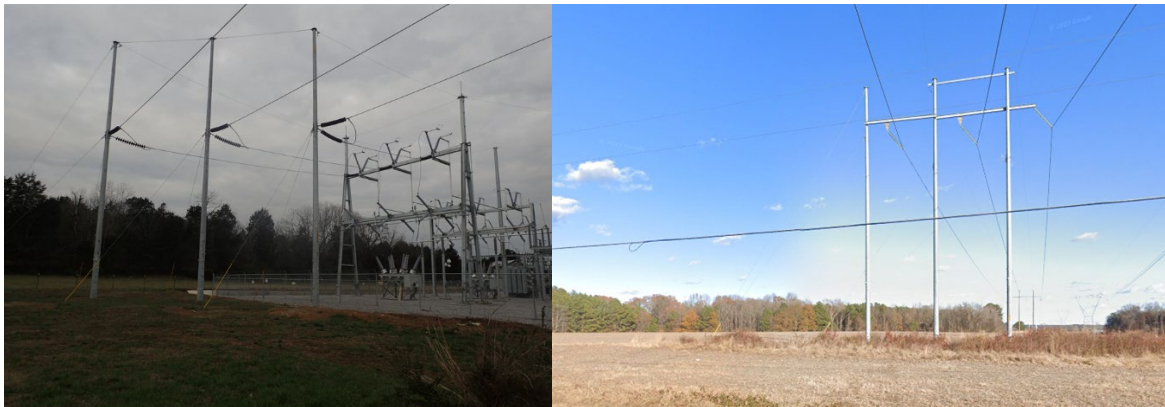
Figure 2-4. Typical Triple Steel-Pole Structures
