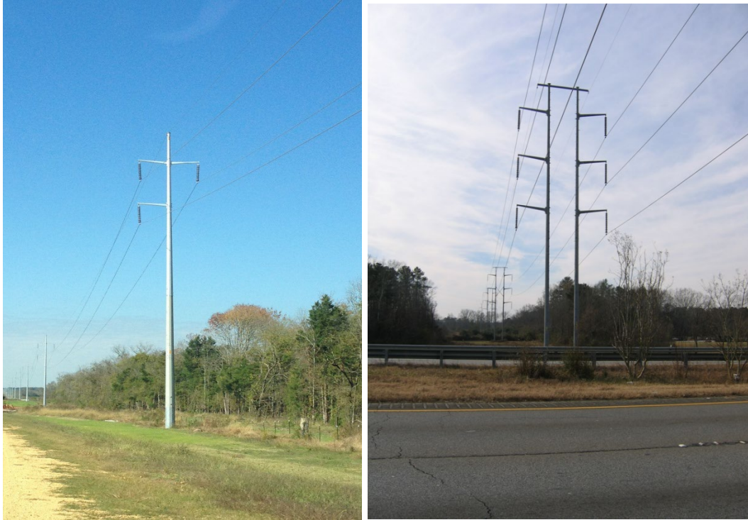
Figure 2-3. Typical Single and Double Steel-Pole Structures
