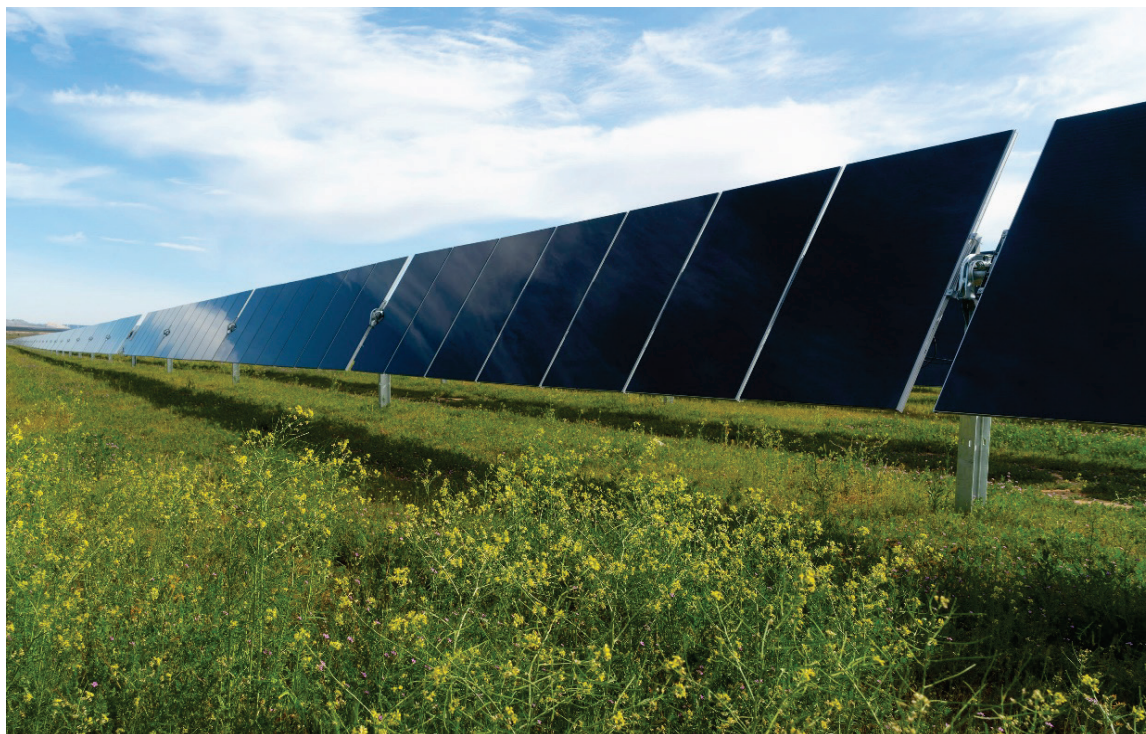
Figure 3-15. Single-axis, tracking PV system with panels near maximum tilt as viewed from the east or west
