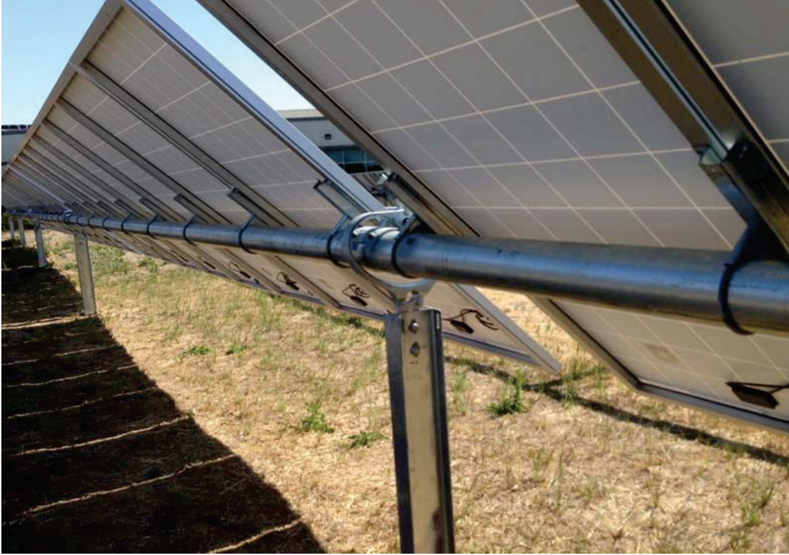
Figure 3-16. The backside of the solar panels in early morning or late afternoon configuration
