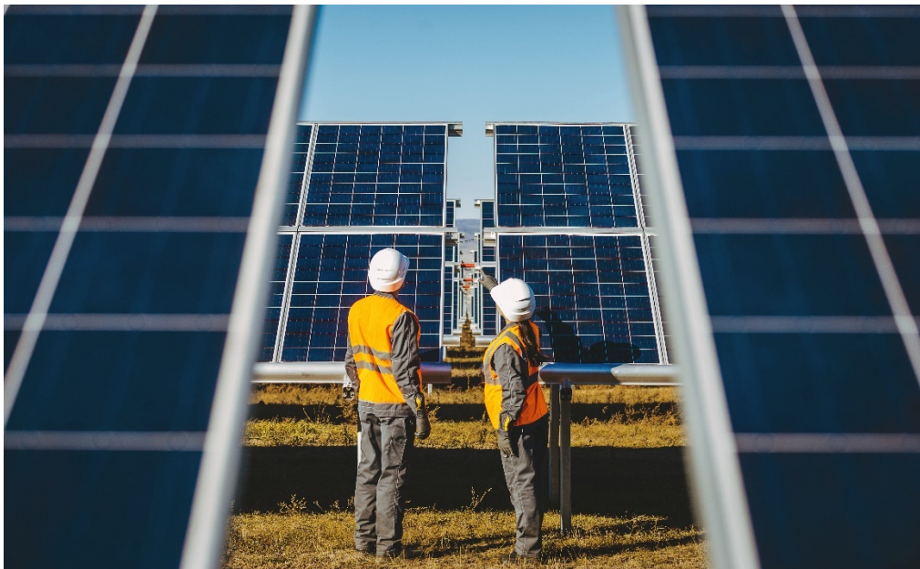
Figure 3-12: Representative Photo of Single-Axis Tracking PV System in the Morning, Facing East
