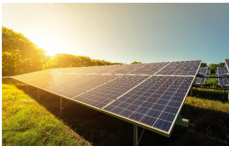
Figure 3-13: Representative Photo of Single-Axis Tracking PV System at Midday, Laying Flat
