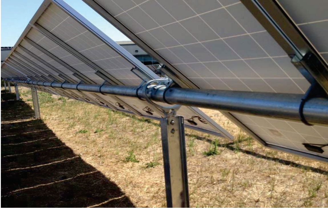
Figure 3-35. The backside of the solar panels in early morning or late afternoon configuration
