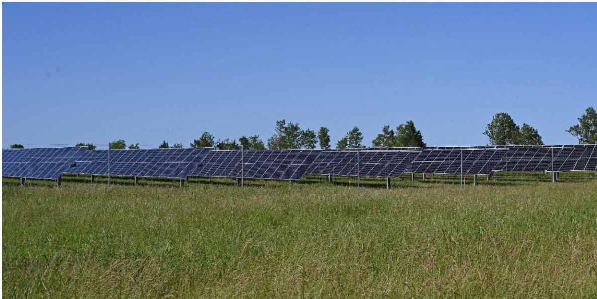
Figure 3-24. PV arrays near max tilt angle.
