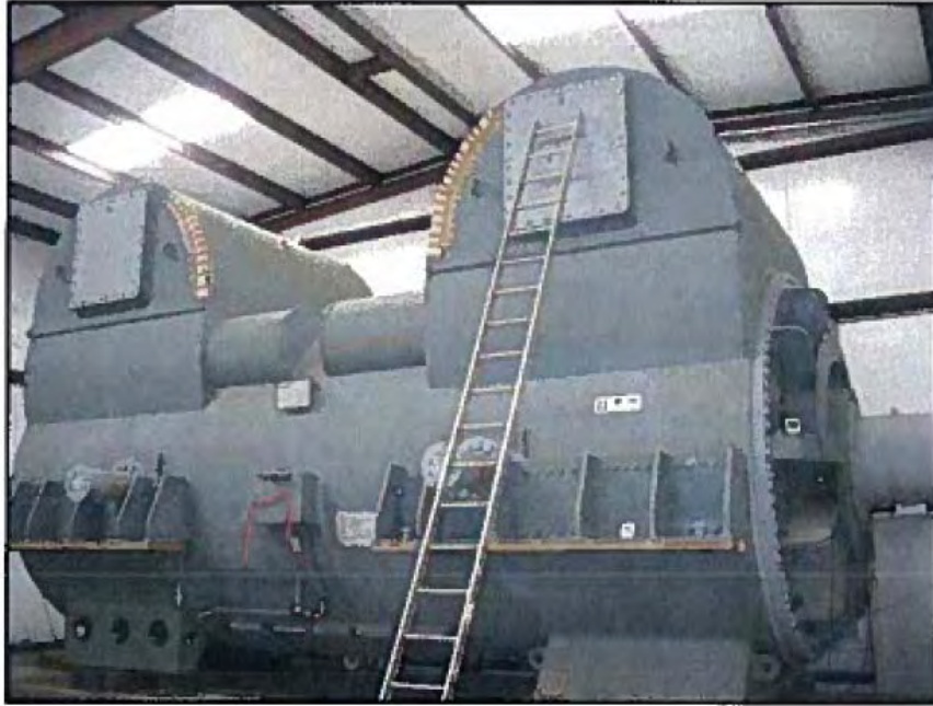
Figure 3-2. Stator Steam Generator
