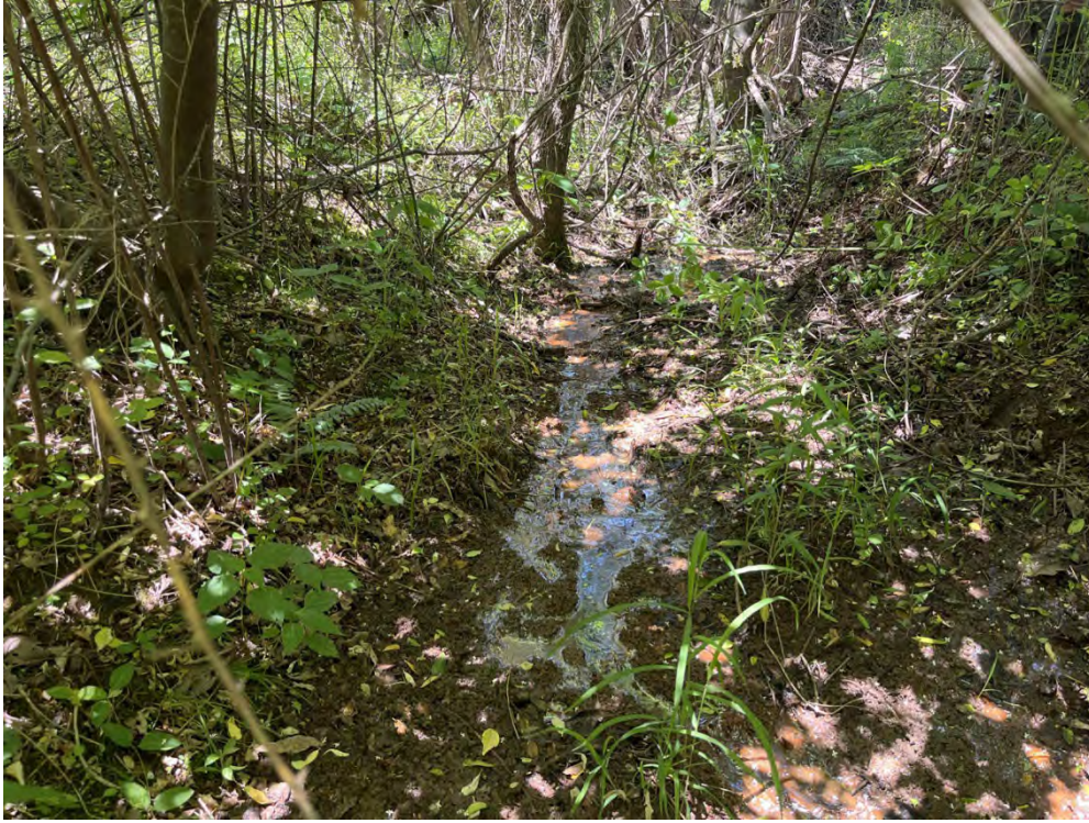
Photo 229. E114, Erosional Gully, facing upstream and northwest.
