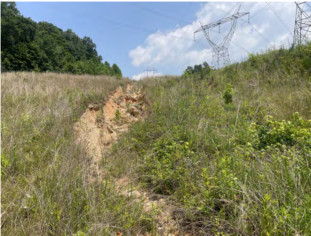
Photo 250. E127, Erosional Gully, facing upstream and north.
