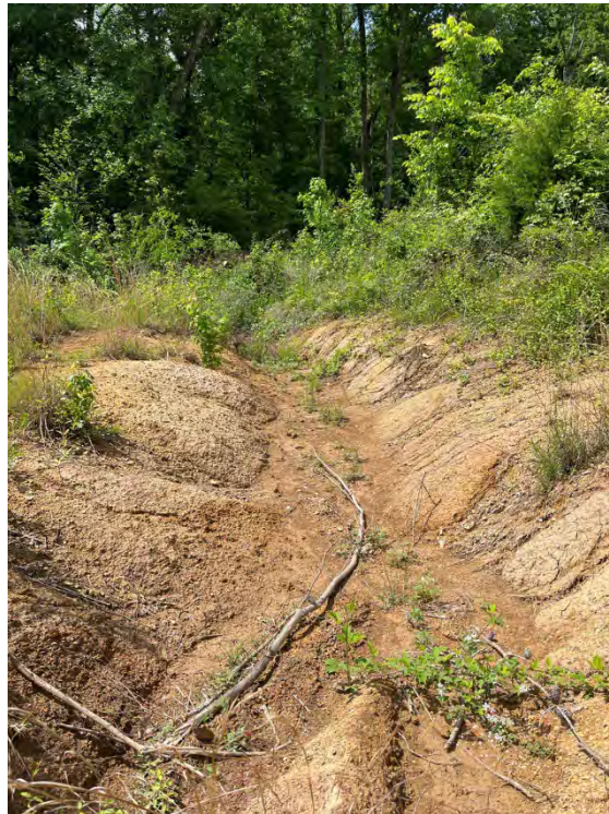
Photo 226. E111, Erosional Gully, facing upstream and southeast.
