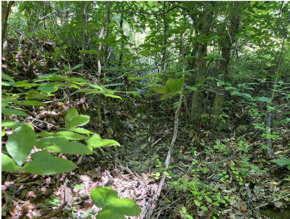
Photo 240. E122, Erosional Gully, facing upstream and northwest.
