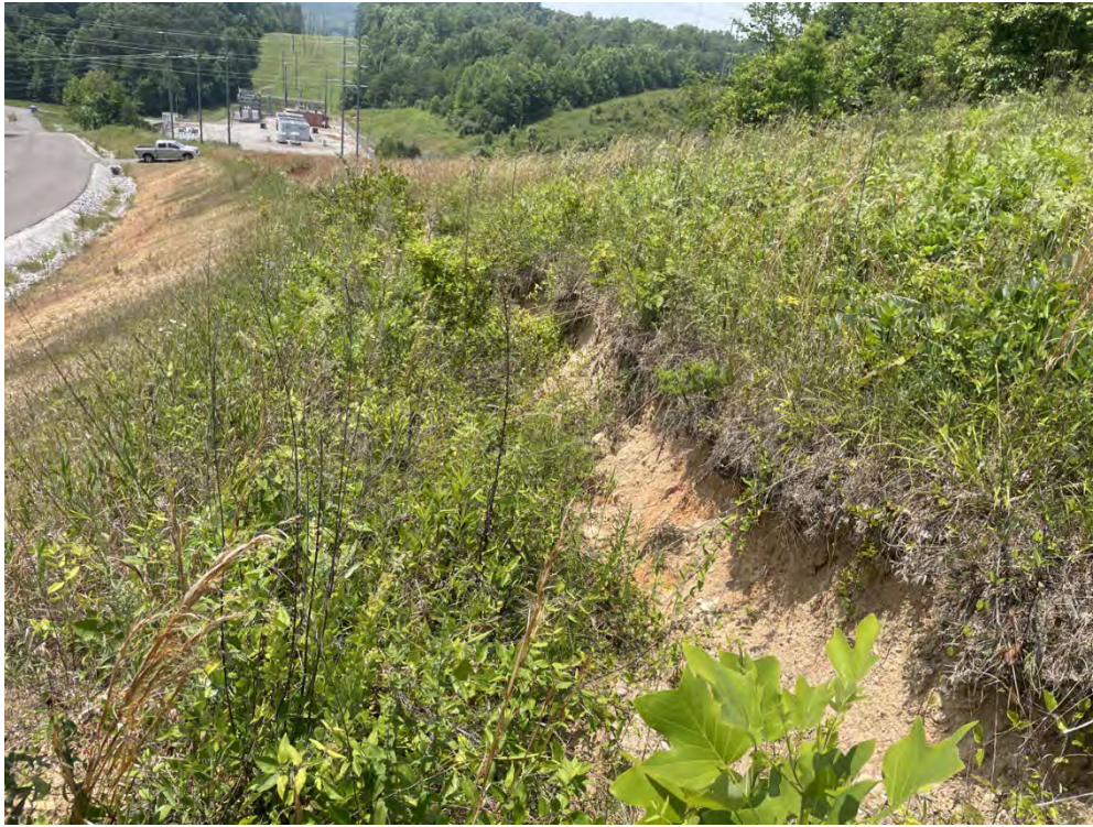
Photo 249. E127, Erosional Gully, facing downstream and southwest.
