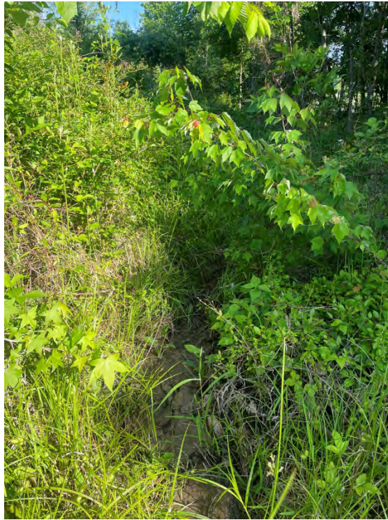
Photo 239. E119, Erosional Gully, facing upstream and northwest.
