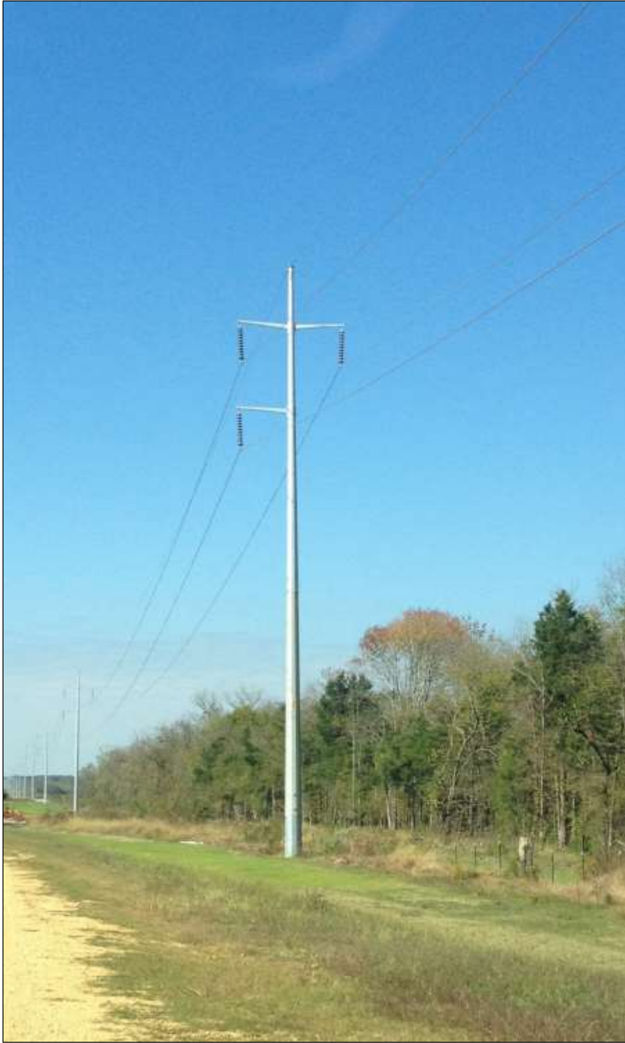
Figure 6. A typical example of the S1G type of steel pole structure (not from the current APE).
