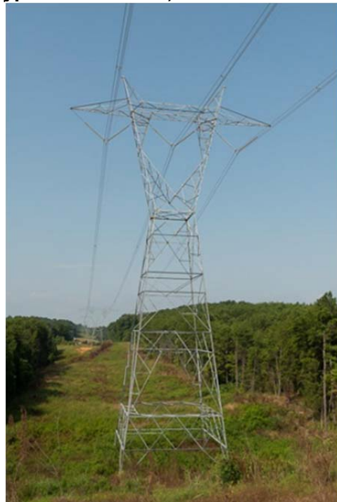
Figure 2-2. Typical 500-kV Laced-Steel Transmission Tower
