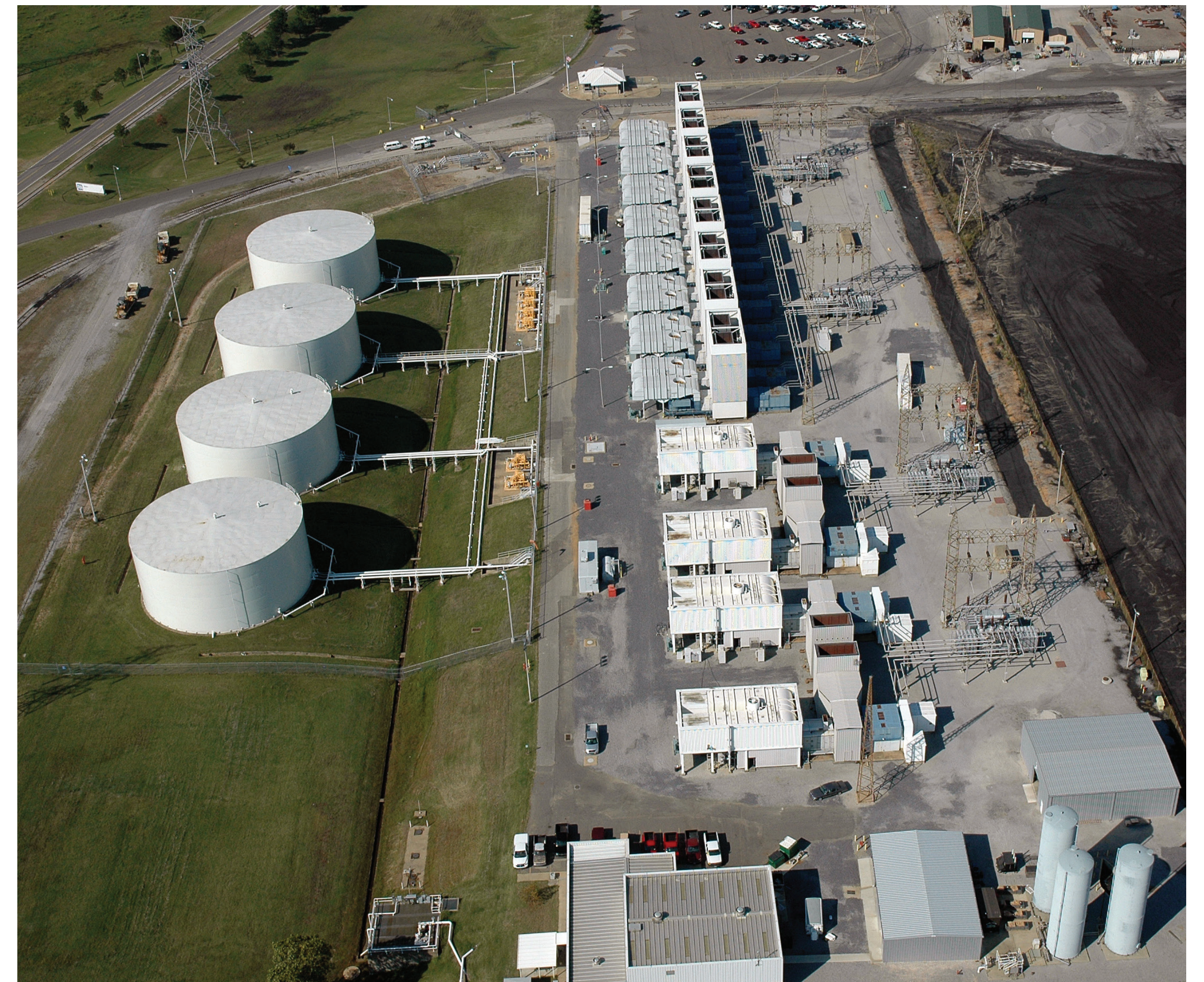
Allen Combustion Turbine Plant
