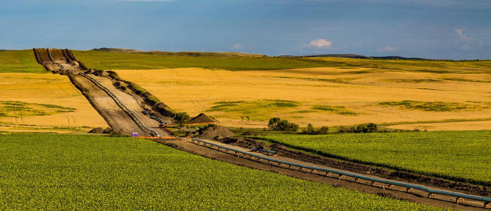
Construction of the Dakota Access Pipeline near New Salem, North Dakota. Tony Webster. (CC BY-NC-SA 2.0)
