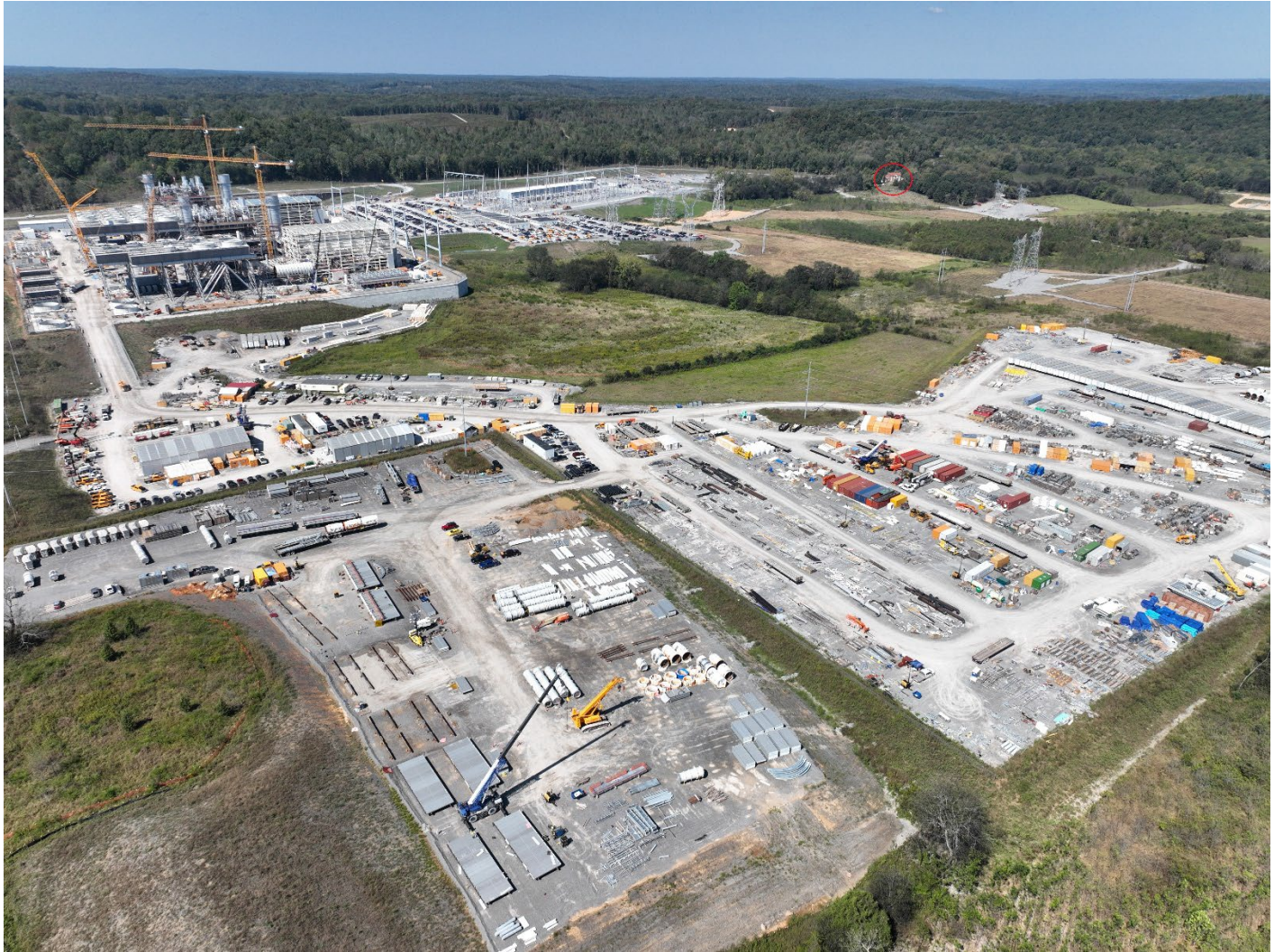
Figure 7 - Photo rendering showing CUG under construction, looking northwest. Existing and planned transmission infrastructure can be seen in relation with SW-745 in the middle of the image (marked with red circle).
