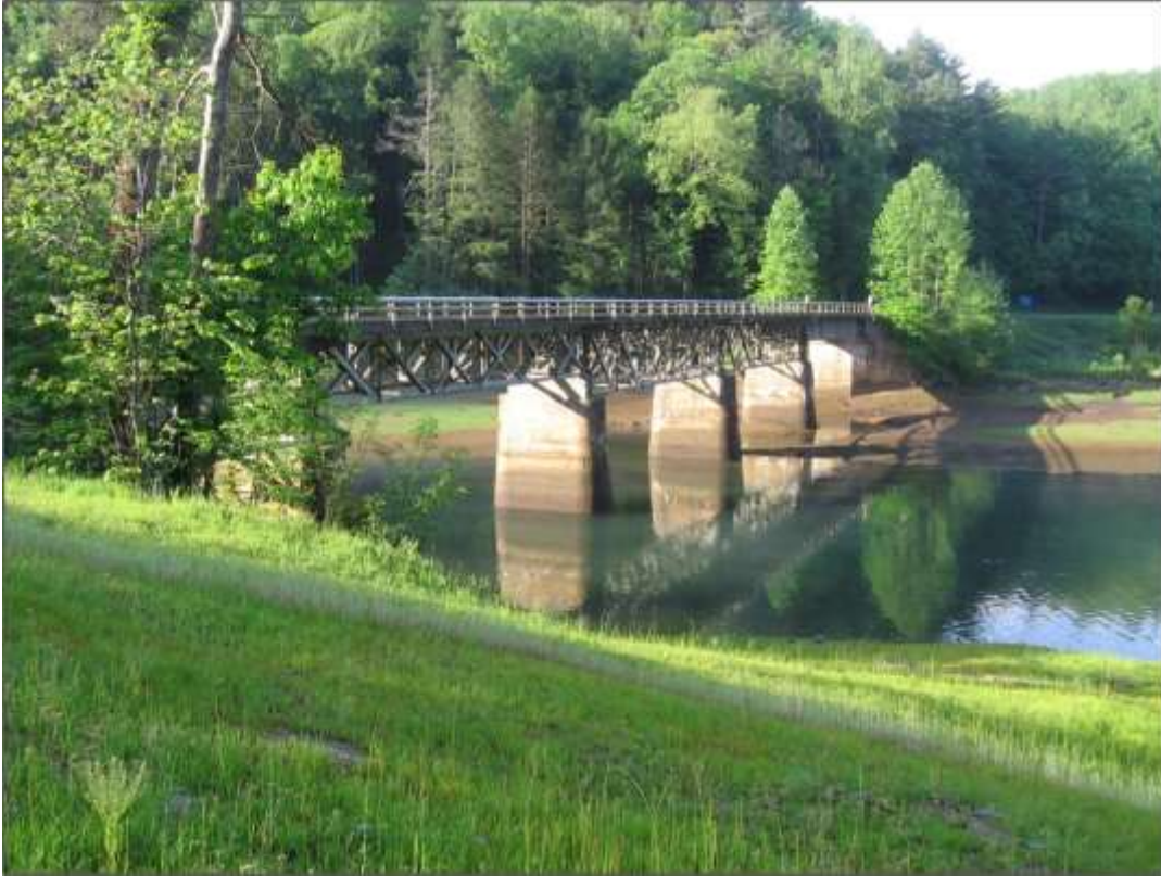
Figure 1. The existing Wilbur Reservoir Bridge, carrying Wilbur Dam Road over Wilbur Reservoir. View to north.
