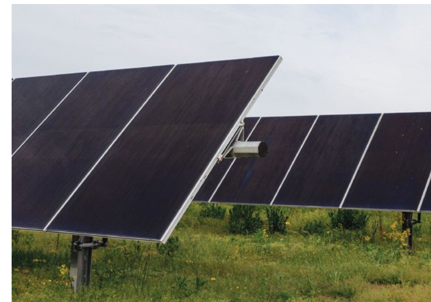
Announced in 2020 and developed under the TVA Green Invest program, Skyhawk Solar contributes to TVA's continued push to grow clean energy in its seven-state service territory.
