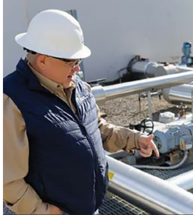
Inspectors check that freeze protection equipment is assembled correctly after every regular maintenance.
