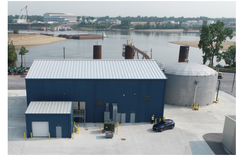
Onsite groundwater pump and treat system
