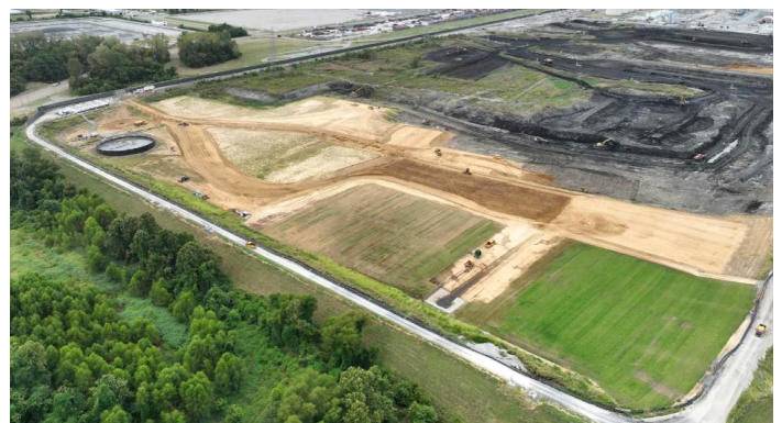
Coal ash removal and site restoration at East Ash Disposal Area is approximately 30 percent complete.
