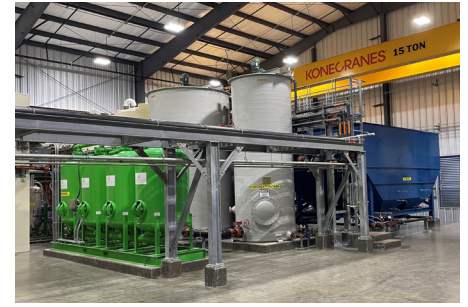
Onsite groundwater pump and treat system
