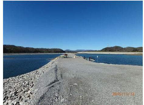
View of Fly Ash Impoundment (Right) and Stilling Pond (Left) along Separator Berm
