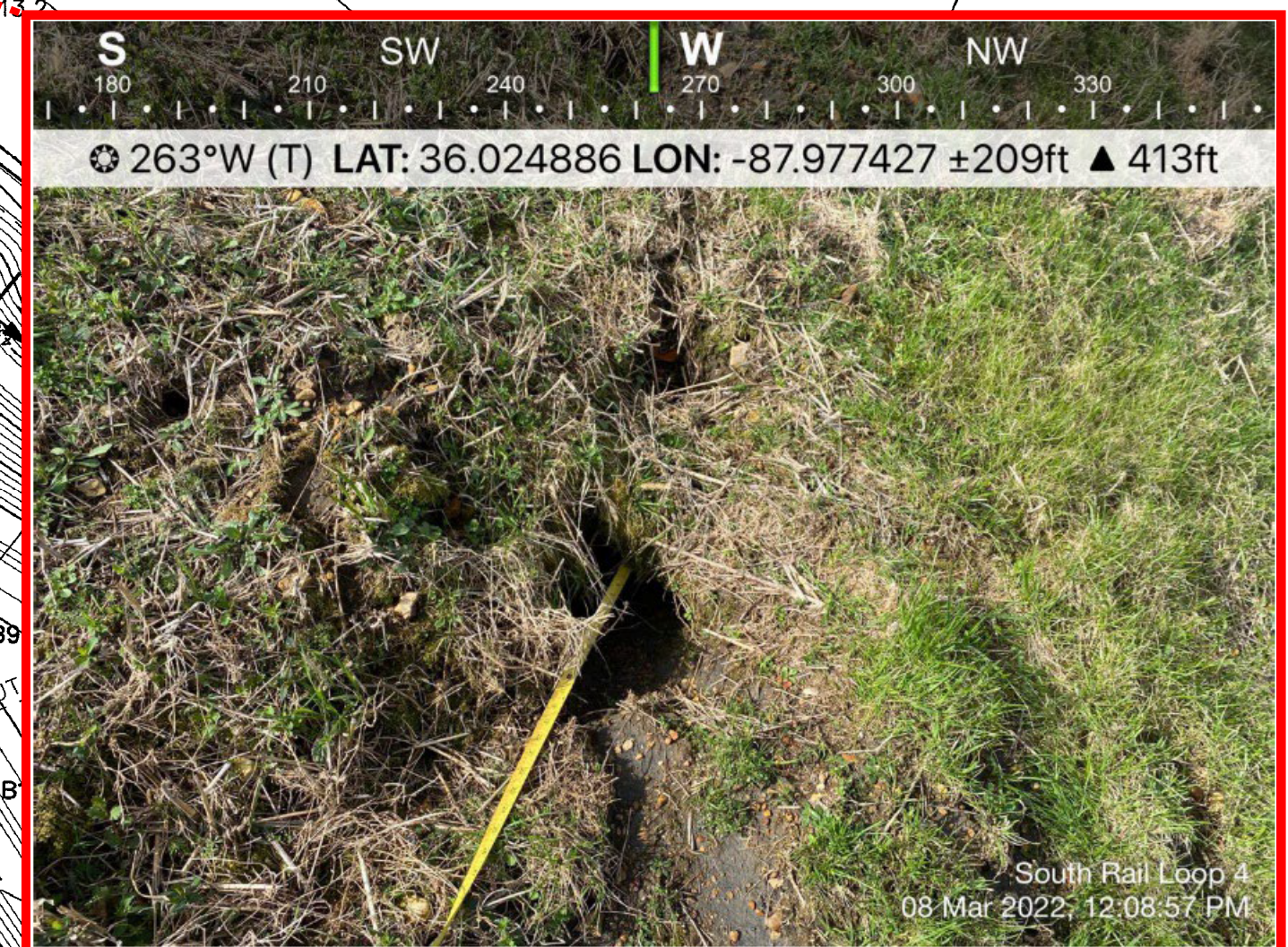
2022 Inspection Report: Photo D-12, "Apparent tension cracking and approximately 20-inch-deep erosion at the northern toe of the South Rail Loop 4 landfill."
