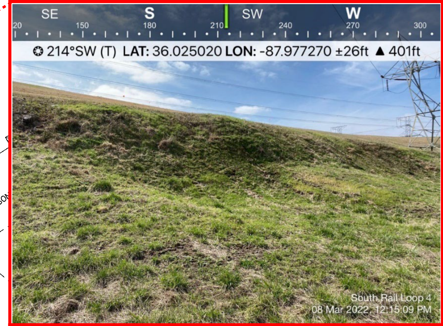
2022 Inspection Report: Photo D-11, "Bulging slope with apparent tension cracking at the northern toe of the South Rail Loop 4 landfill."
