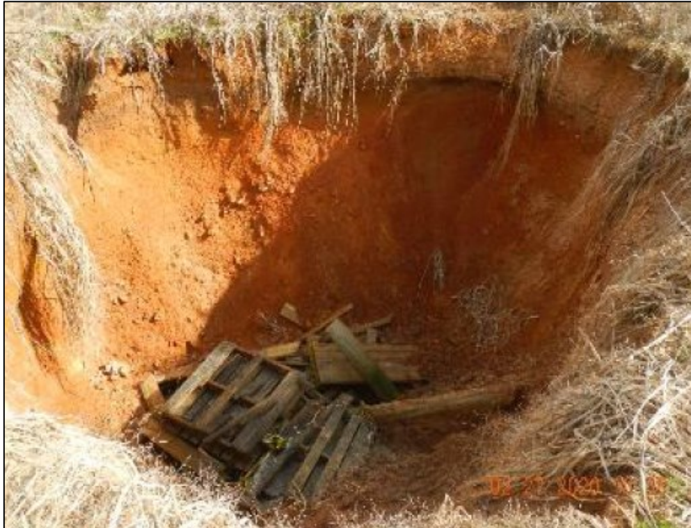
Figure 3.7 Representative Photograph of Sinkhole Feature Encountered During Karst Survey
